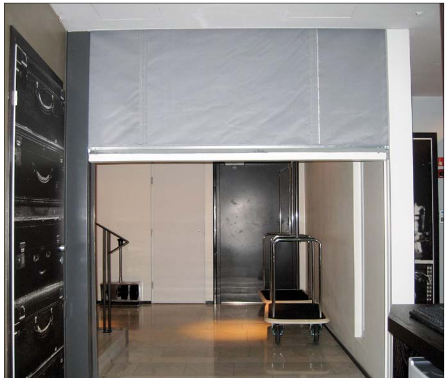
Roll-down fire door installed in a hotel corridor.
